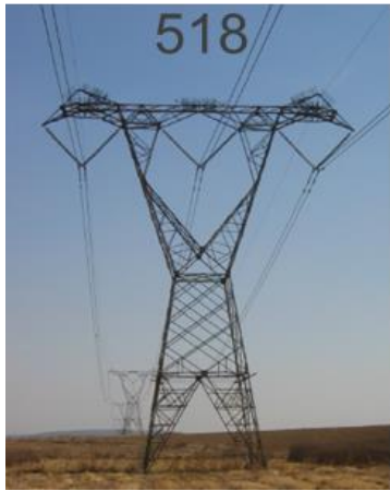
518h: Self Supporting Suspension Tower
