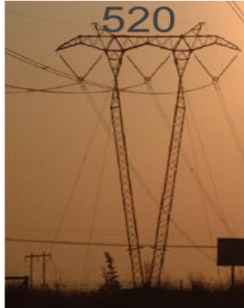
520b: Guyed-V Suspension Towers
